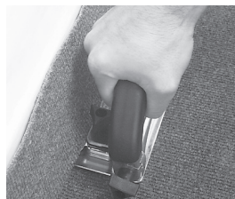
2. Keeping the base plate flat on the carpet and the guide bar against the wall, make the trimming cut.
